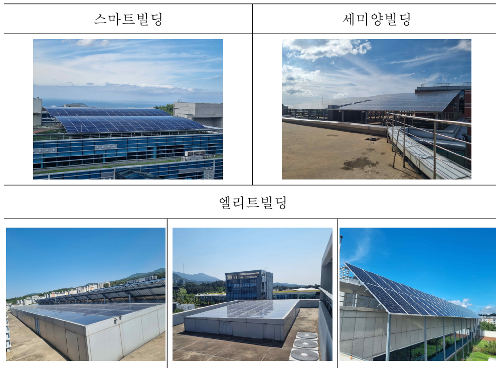
Fig. 7 PV systems on the roofs of three buildings in the Jeju Science Park
