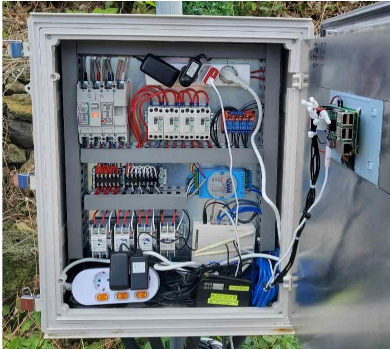
Fig. 14 Irrigation control system of demonstration site #1
